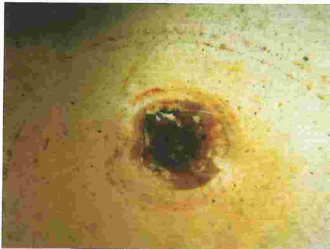
PERFORATIONS IN FLOOR PLATE (REPAIRED WITH EPOXY)
