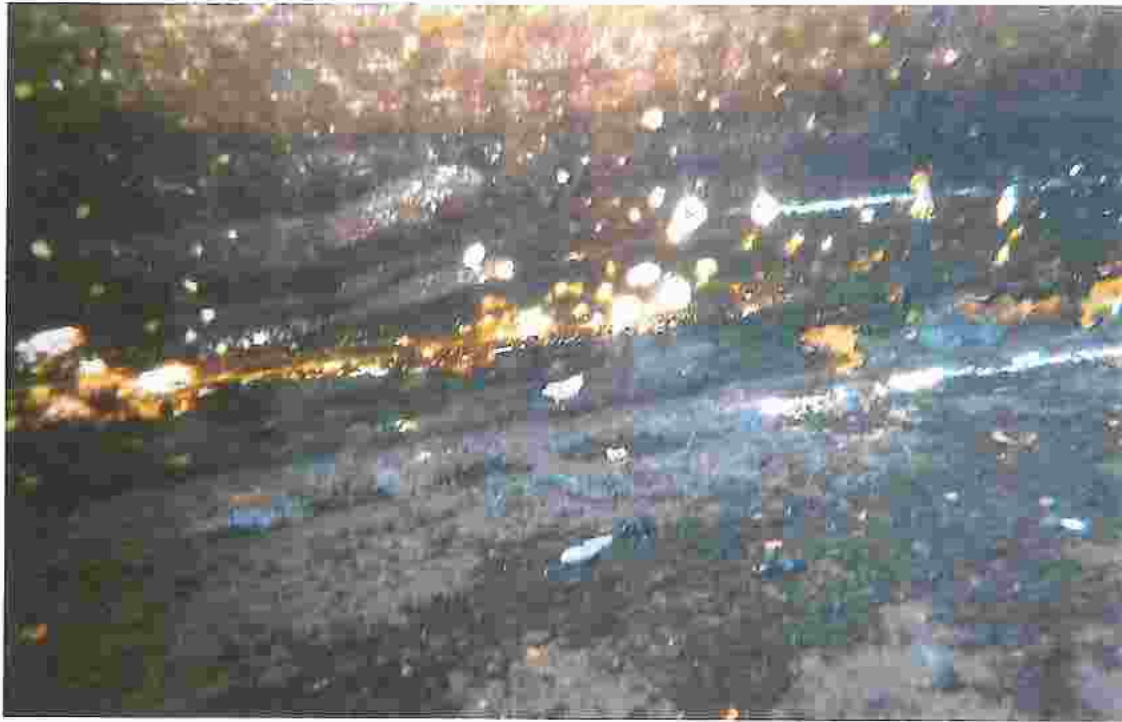
PINPOINT RUST ON LOWER SHELL
