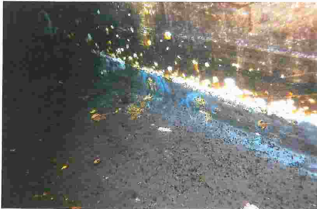
PINPOINT RUST AT LOWER SHELL
