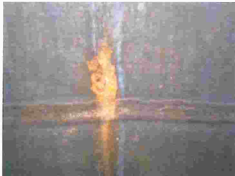
SPOT AREA OF MINOR SURFACE CORROSION ON SHELL
