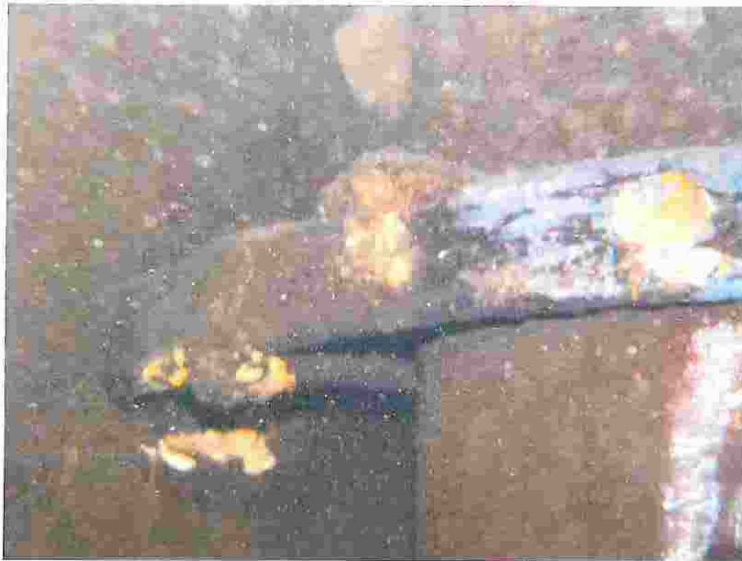
WATER PIPE SUPPORT BRACKETS
