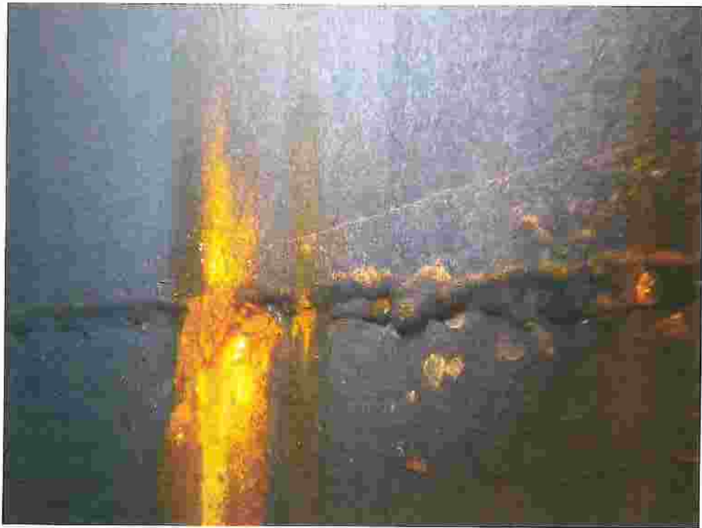
SHELL SURFACE MINOR CORROSION
