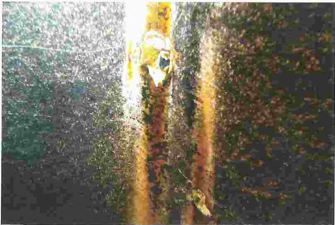
MINOR SURFACE RUST ON SHELL WELD SEAM
