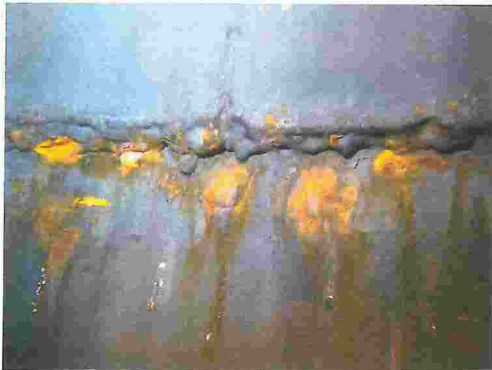
SHELL WELD SEAM WITH MINOR SURFACE CORROSION
