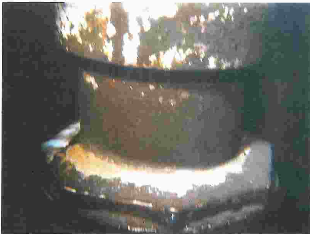
STEEL PIPE TO PVC ADAPTER ON INLET WATER PIPING
