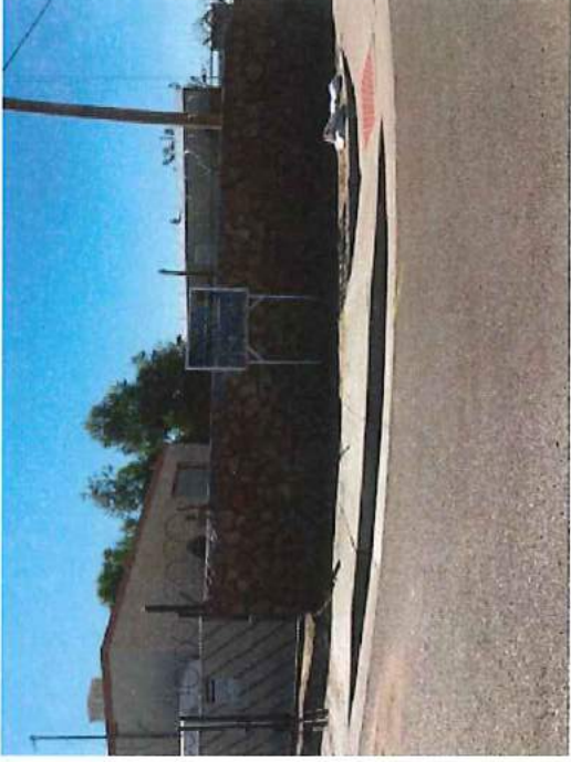
Elks Drive Booster Station 1 acre est.
